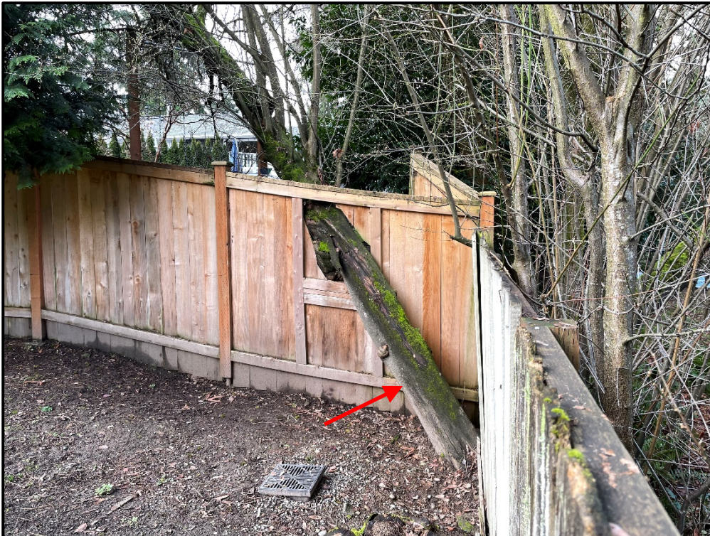
Photograph 2. Photo taken looking over the fence on the southern property line. The south trunk of tree 214 is indicated by the red arrow.
